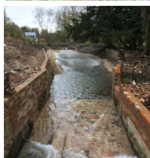
Looking u/s. Structure removed, historic brick work made good. Passable for fish, upstream silt removed. 300m of channel restored.
