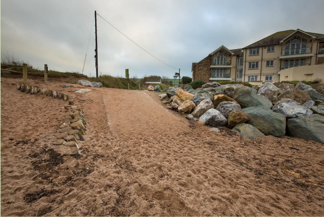
Photo 2: Slipway (National Trust) and rock revetment (not National Trust) (source: Robert Harvey)
