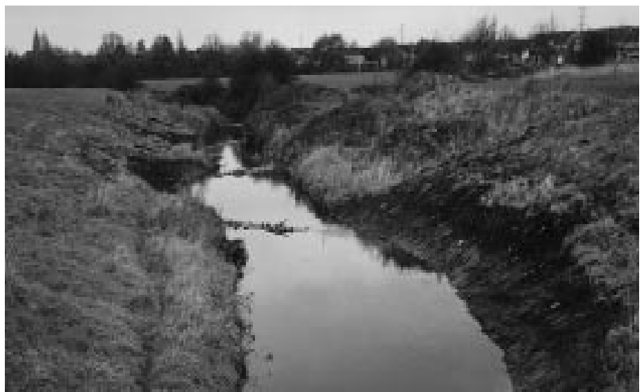
Where the channel has not been moved, bays have been dug downstream of groynes to encourage the river to use its own energy to create meanders.
