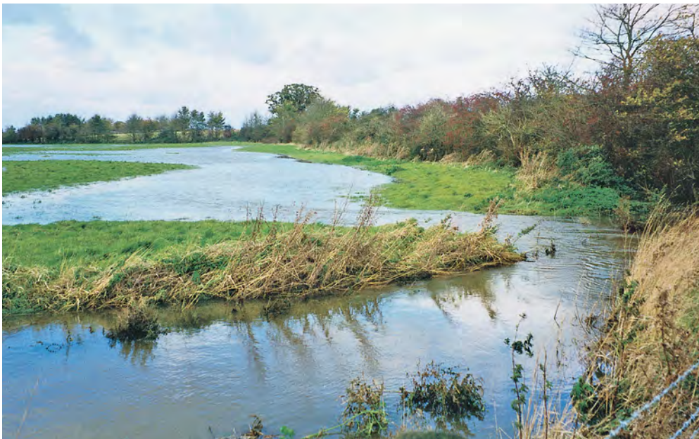
Spillway S4 . Floodwaters spilling into field gully.
