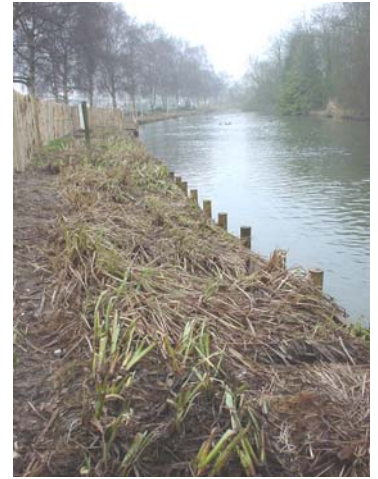
Coir mattress bank revetment on the Wensum, Fakenham. Temporary fencing erected to allow structure to stabilise
