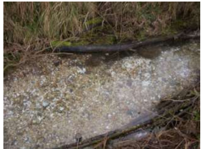
Freshly placed gravel and chalk mix. Faggots are partially hidden and large woody debris is placed to give a more natural appearance.
