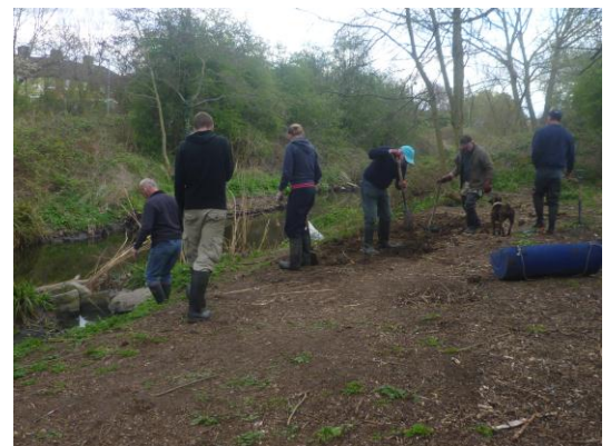
Thames 21 volunteers helping to backfill a side berm on the left bank of the River Pool
