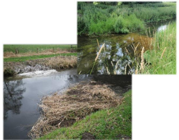
Double shoulders under construction (left, with far bank berm yet to be capped), and 4 months later (right). © 2010 Nigel Holmes and 2011 Chris Bell
