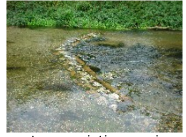
An upstream pointing v weir made from logs obtained locally with large cobbles placed upstream
