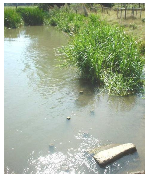
View of one of the sections where the coir rolls have been washed away, leaving the stakes behind
