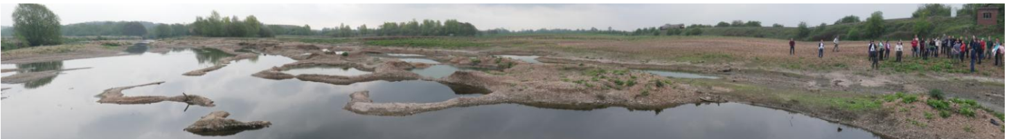
View of some of the complex micro-topography created in the widest part of the works. © 2011 The River Restoration Centre
