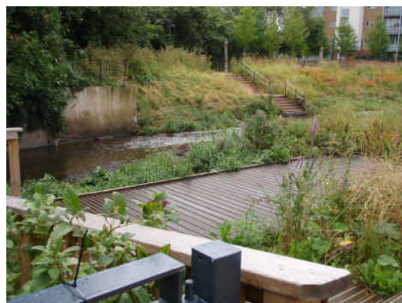
River Ravensbourne following removal of concrete channel and provision of board walks
