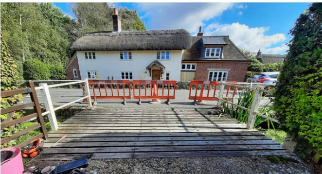
Before: The weakened bridge
