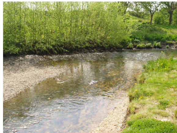
Bank stabilisation with crushed concrete (hidden) and live willow poles providing good marginal habitat
