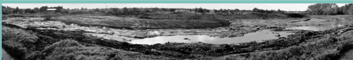
Corridor excavated and low flow channel form established. Note current brook is not connected. (October 2004)
