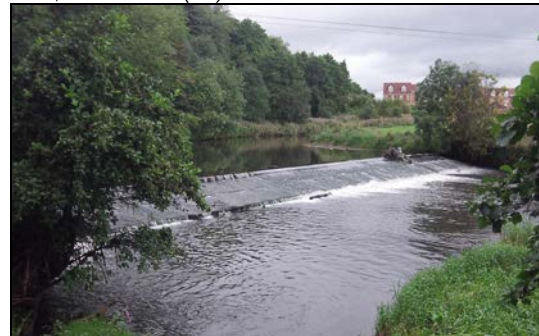
Before removal of weir: photo courtesy of Oliver Southgate, Environment Agency (UK)
