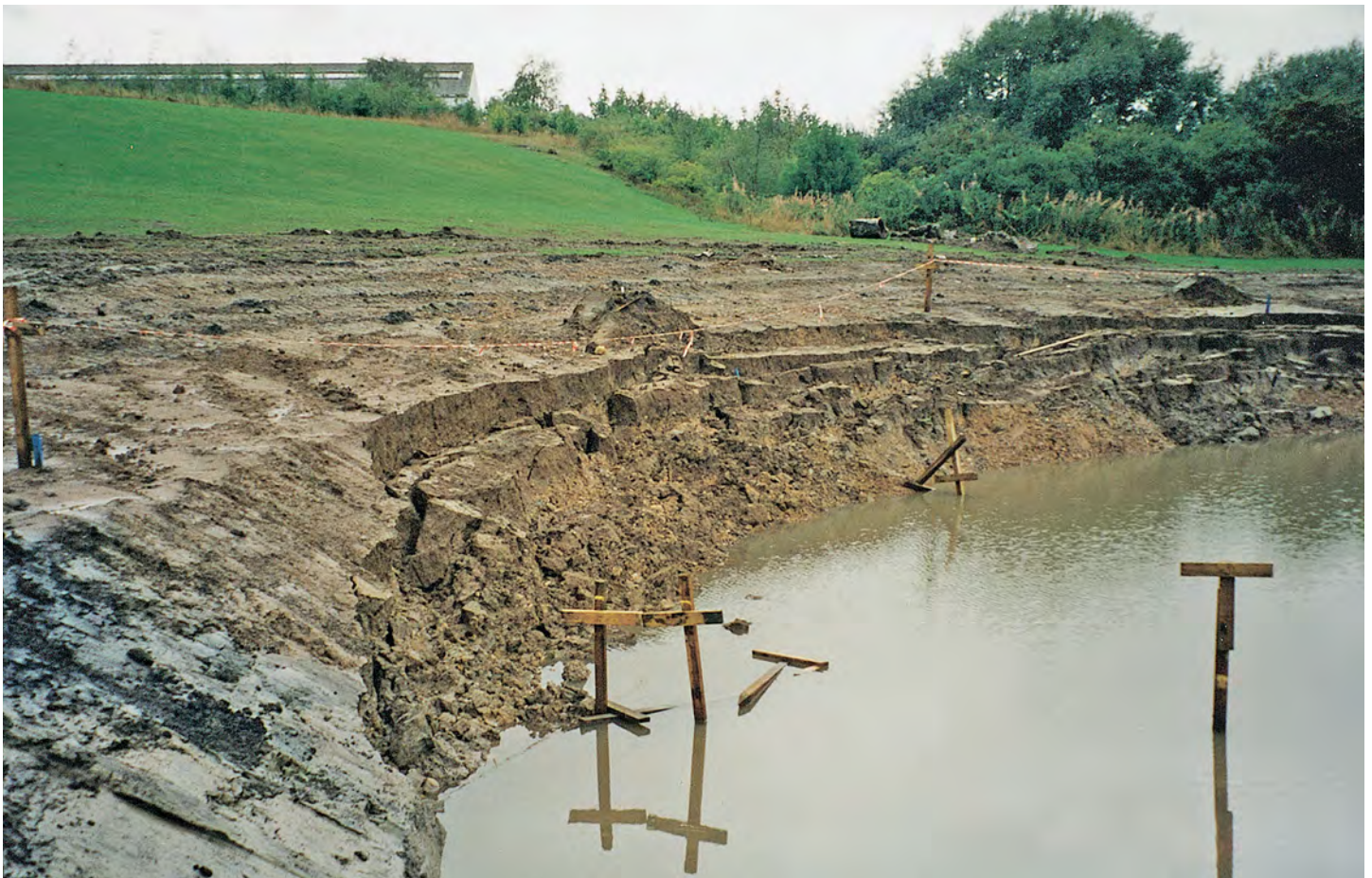
Slipped slope during work – September 1995
