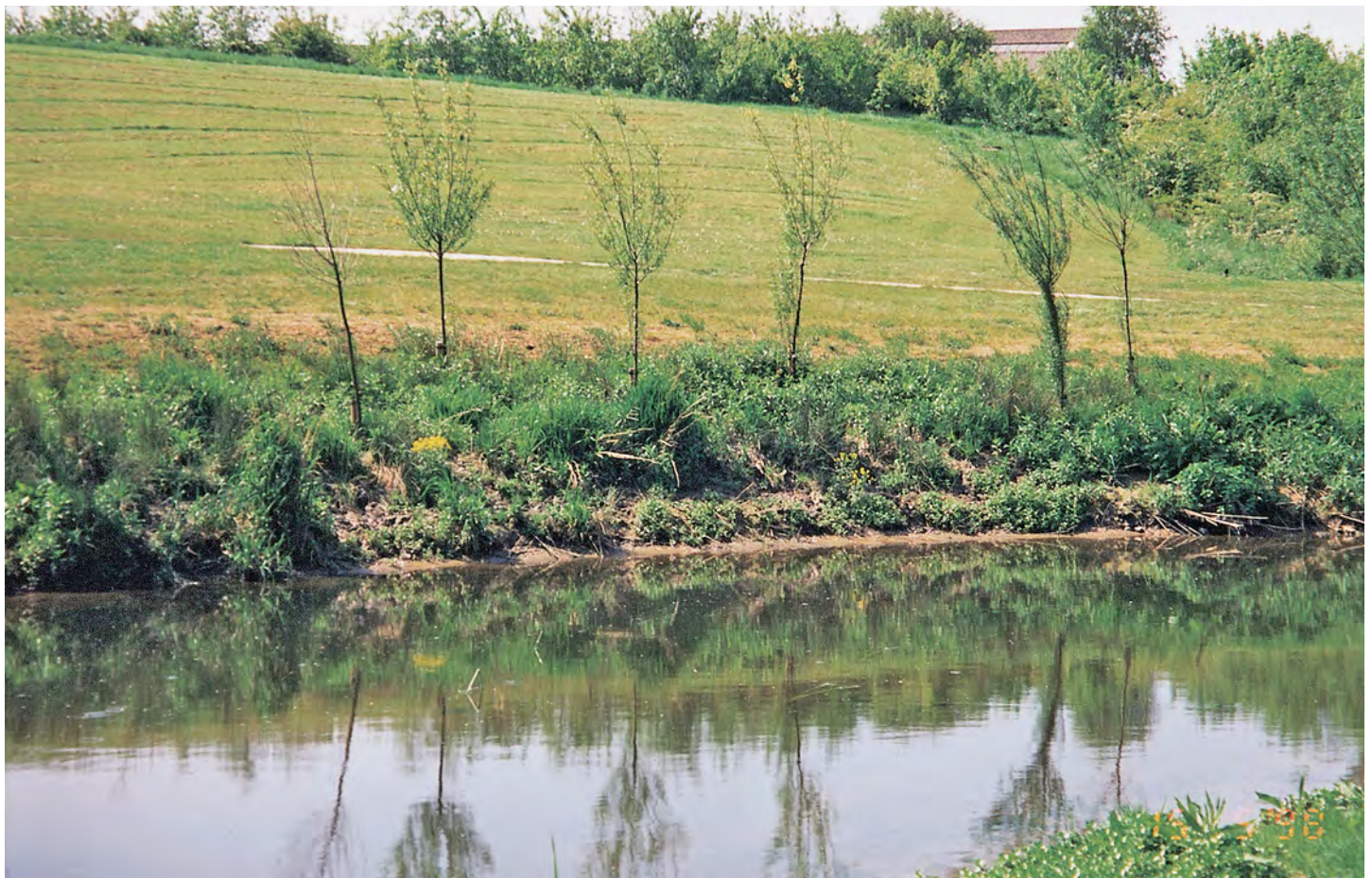
Slipped slope 2 years after repair – 1997
